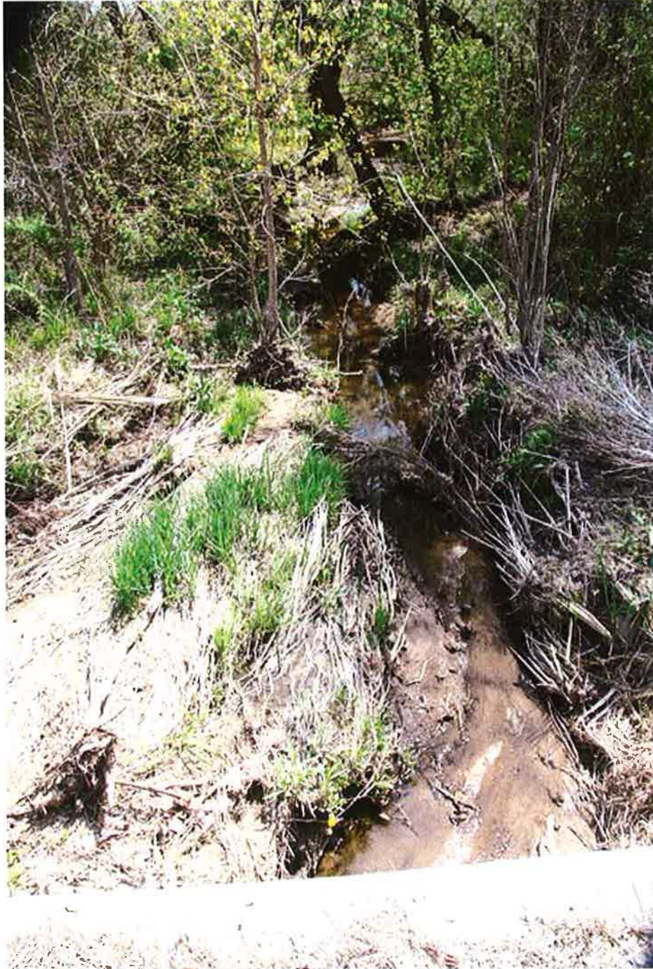
Site US51-68. Unnamed tributary (e) of Vandalia Lake, at the Illinois Route 185 box culvert, 3.7 mi (6.0 km) SW Vera (town). Looking downstream / south. Photo by M.J. Wetzel, 14 April 2011. [ an upstream photo precedes this one ]
