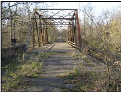
Multiple alternatives were developed where US 51 crosses Ramsey Creek, including an alternative that utilized the corridor sharing the bridge carrying Old US 51 over Ramsey Creek.
